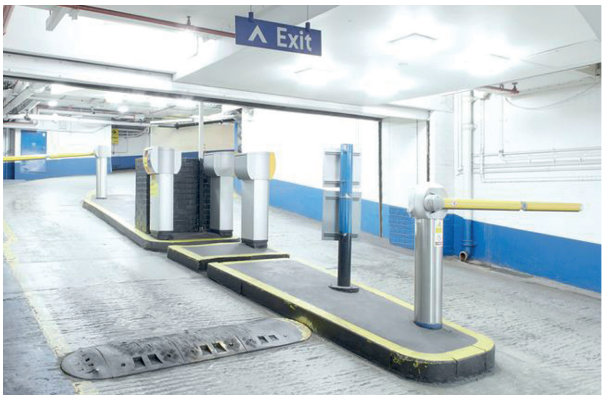
01 Example of use within a car park
