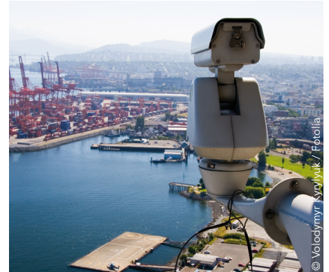
Building Automation & Control
